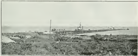
Hudson Bay Terminus. Government pier, showing temporary trestle. The locomotive crane in the centre of the picture is driving piles for bridge seats. Native timber is shown in the foreground.
