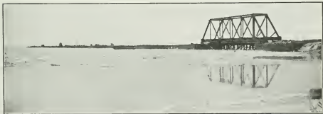
Hudson Bay Terminus. General view of pier in latter part of October, showing the erection of first span of bridge nearly completed. The remaining spans will be erected by the cantilever method.
