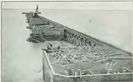
Hudson Bay Terminus. View looking towards ship channel, showing work in progress on bridge piers. In the foreground hardwood and steel plate ice protection is being placed. In the immediate foreground, piles for the support of steel superstructure may be seen.
