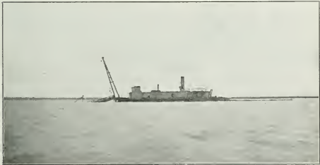
Hudson Bay Terminus. Hydraulic dredge "Port Nelson" at work in the ship channel.
