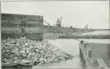
Hudson Bay Terminus. View from season's terminal crib, looking shoreward, showing riprap protection about piers.
