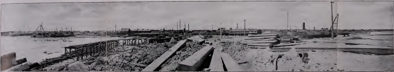
Hudson Bay Railway Terminus at Port Nelson. View from end of Breakwater in early Spring.
