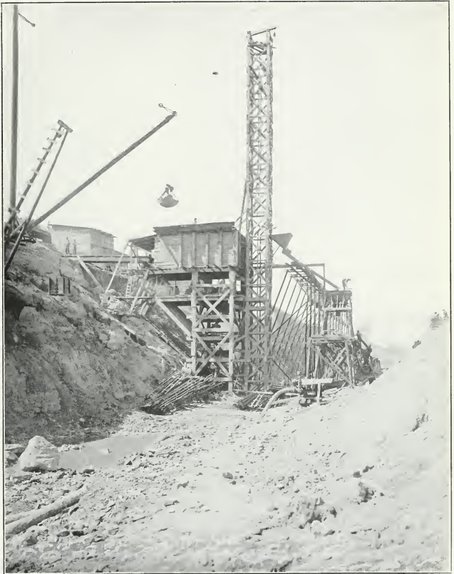
New Welland Ship Canal. Mixing plant and steel reinforcement for concrete entrance wall, Lock No. 1.
