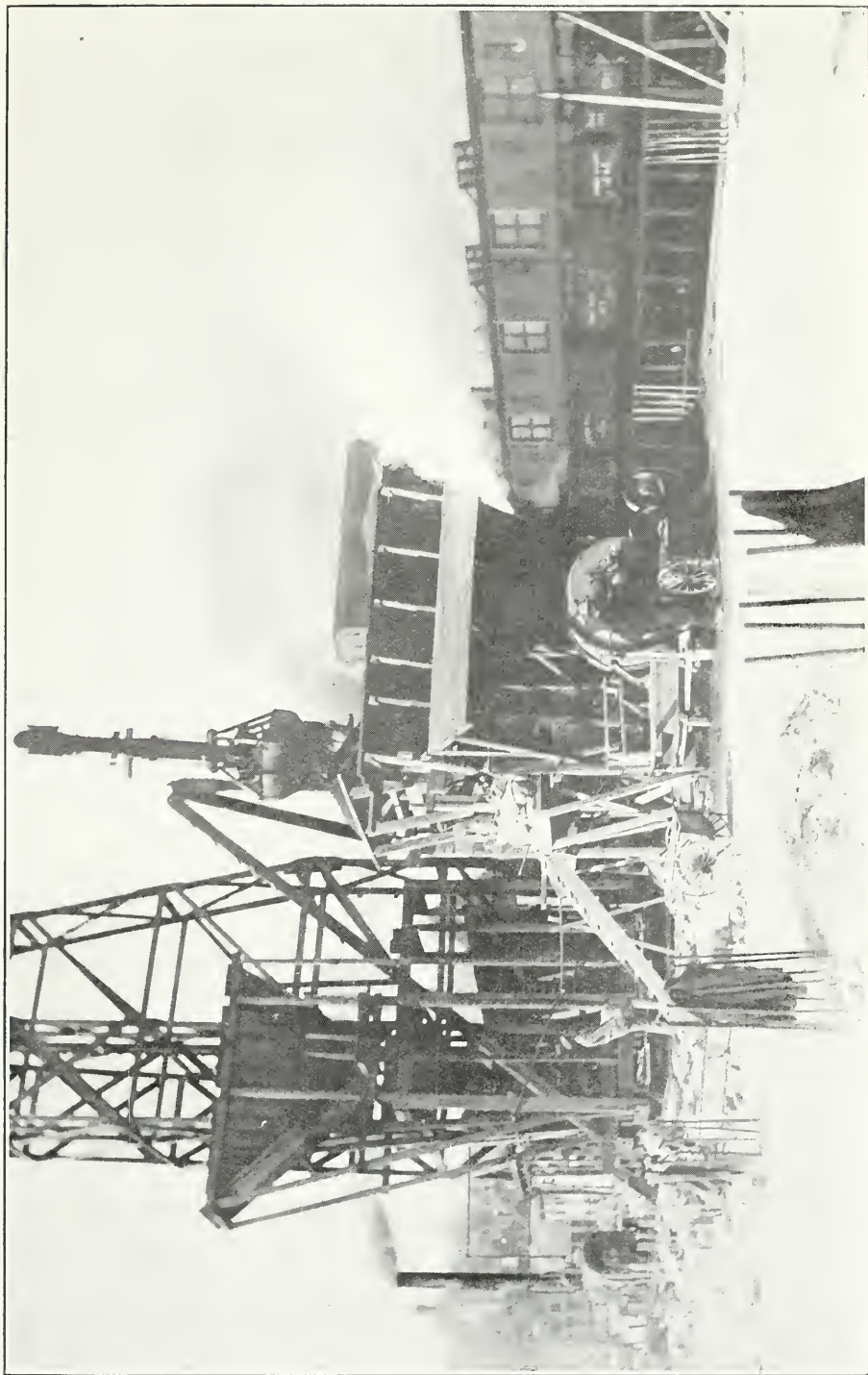
I. C. R. Halifax Terminals—Concrete mixing plant.
