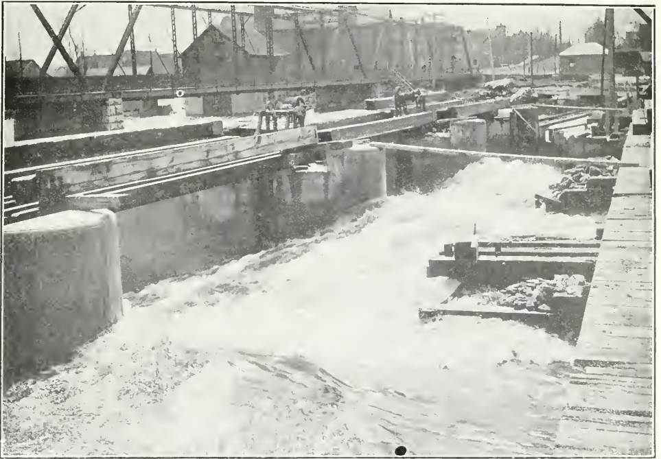
Trent Canal—Ontario—Rice Lake division, new dam at Hastings from north end of old dam.
